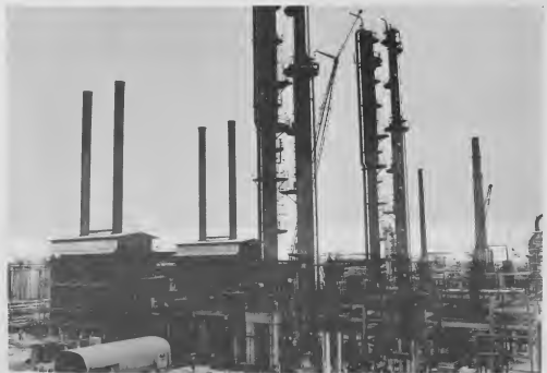
The two new Hydrogen Plants, situated north of Powerhouse No. 1, are far advanced on Oct. 1, 1970.
